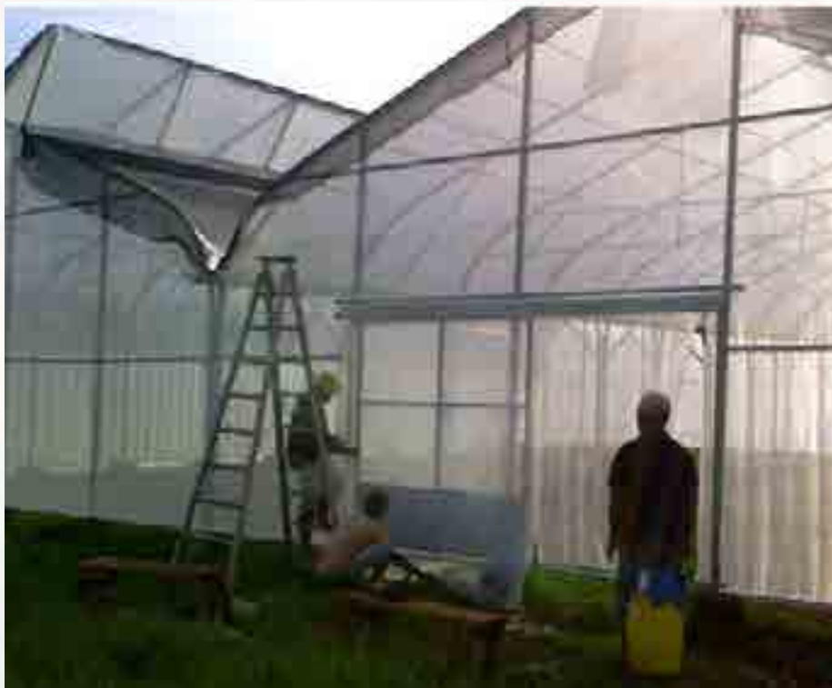
The taller ventilated structures will help trellis crops such as tomato to higher levels thus increasing production with more harvests throughout the season.
